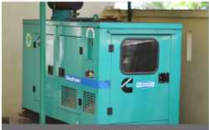
Power Back up
